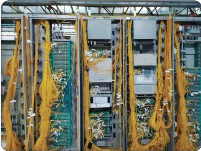
ODF Termination - Before (Patch Cord with fixed length)
