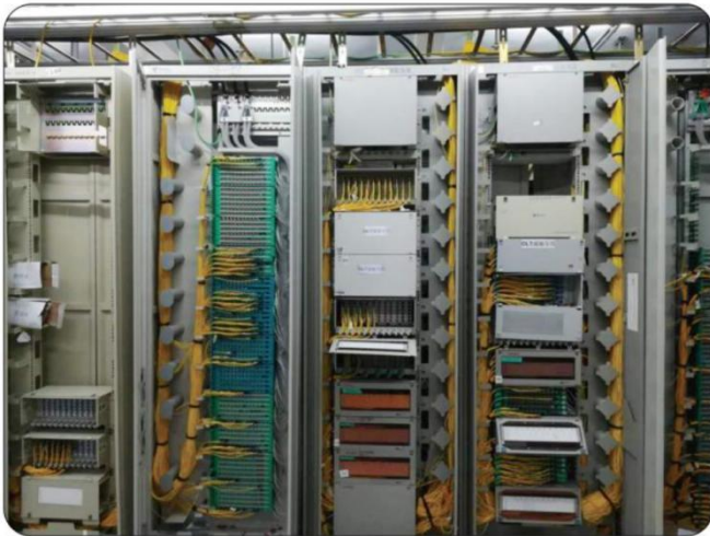
ODF Termination - After (Patch Cord with flexible length)
